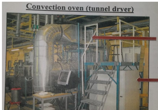
Figure 3: Convection oven (Tunnel dryer)
